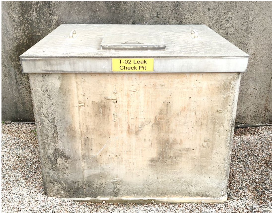
(29) Collection chamber located adjacent to tank foundation is maintained in good condition with periodic inspection
