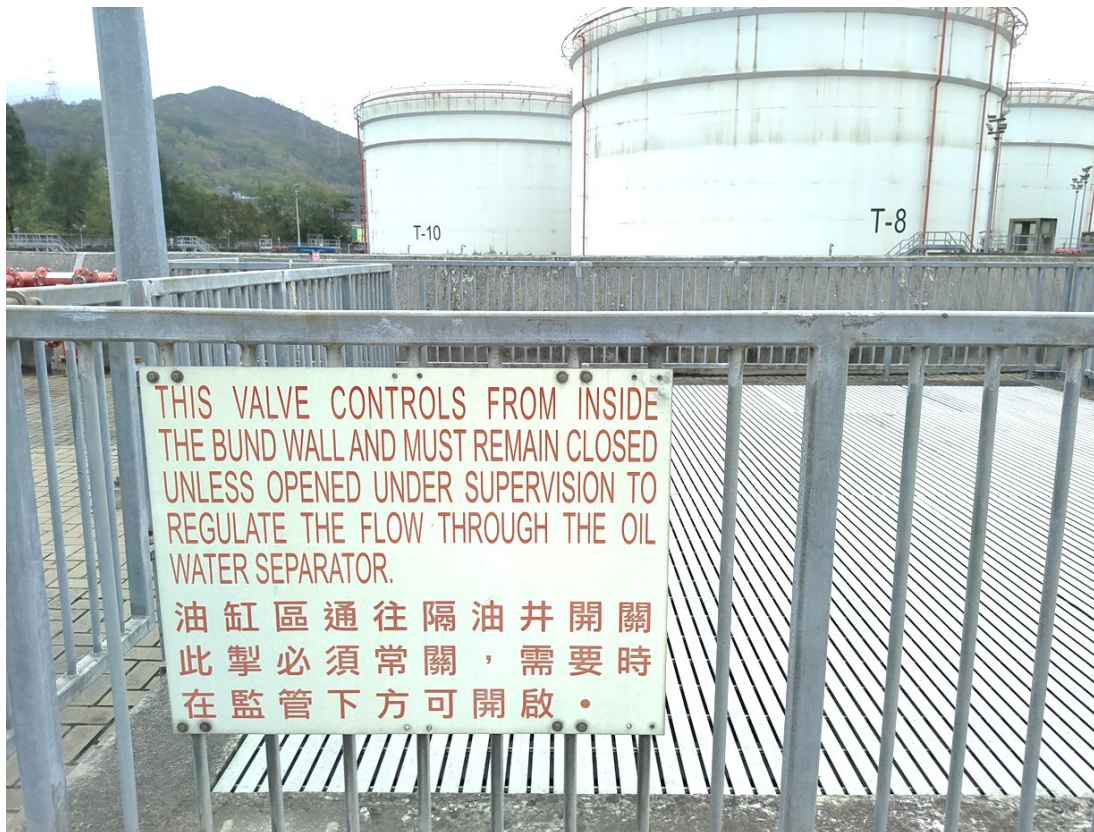
(21) Outlet valve provided for Phase 1b Interceptor with instruction sign to keep “normally closed”
