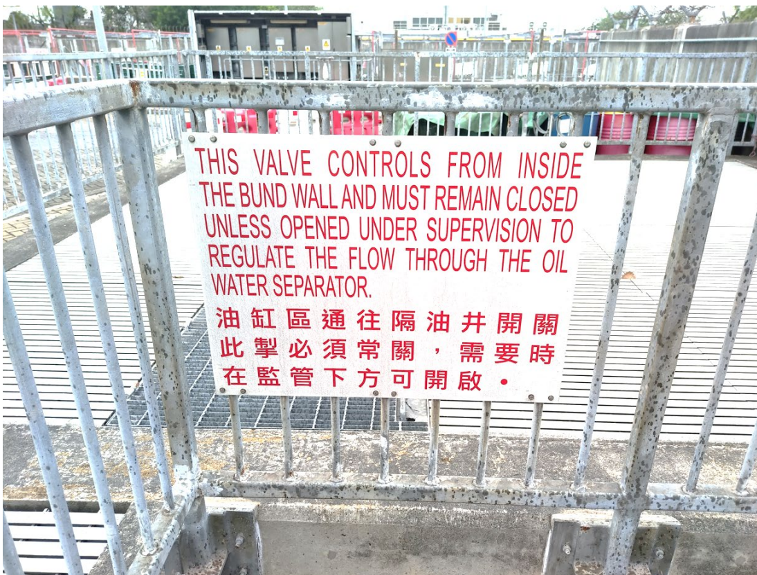
(20) Outlet valve provided for Phase 1a Interceptor with instruction sign to keep “normally closed”
