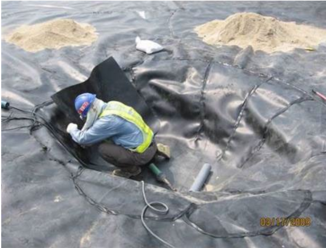
(23) Record photo shows imperious membrane laid at tank center sump with tell-tale pipe embedded for leak detection
