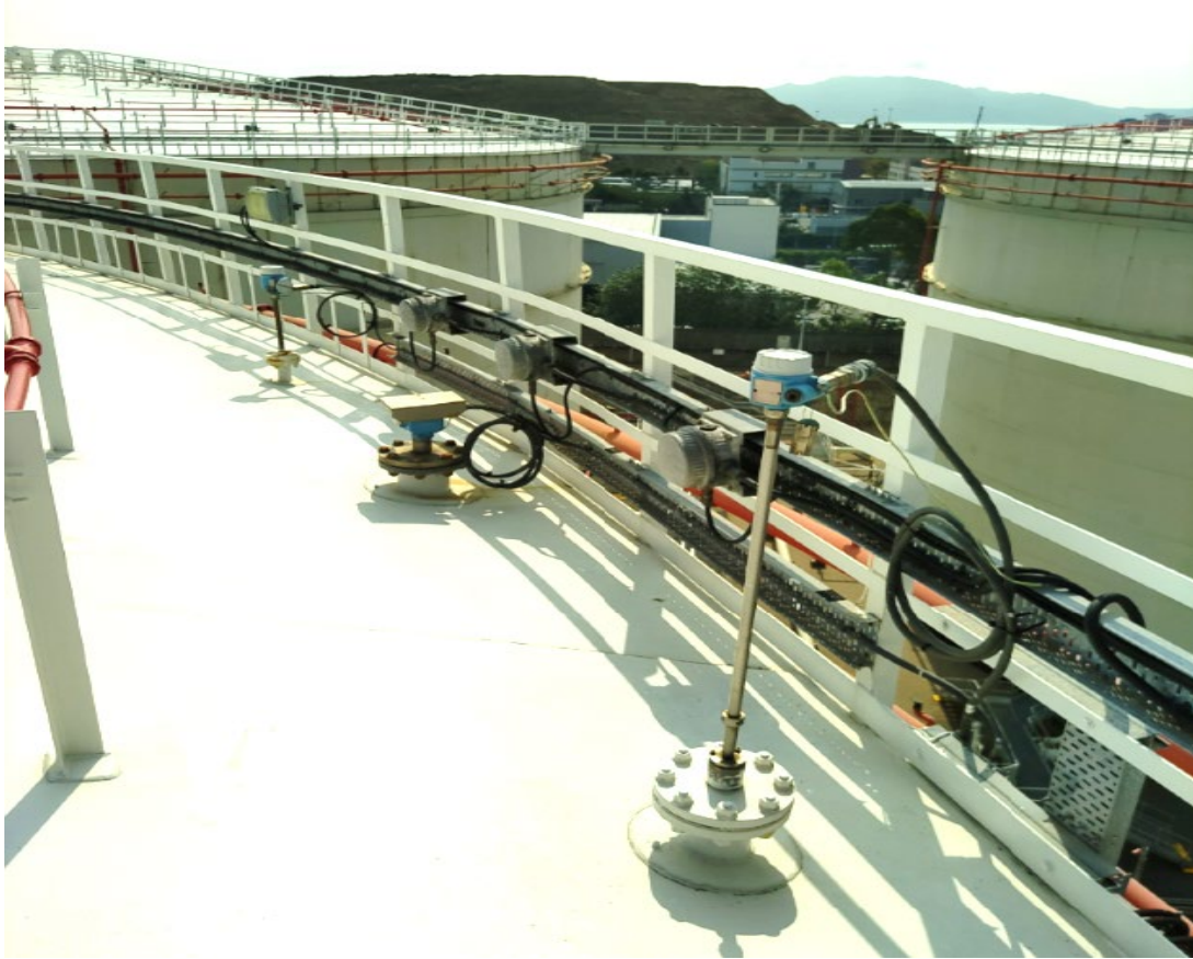
(25) Regular inspection performed on overfilling monitoring device (High-High Level Alarm)
