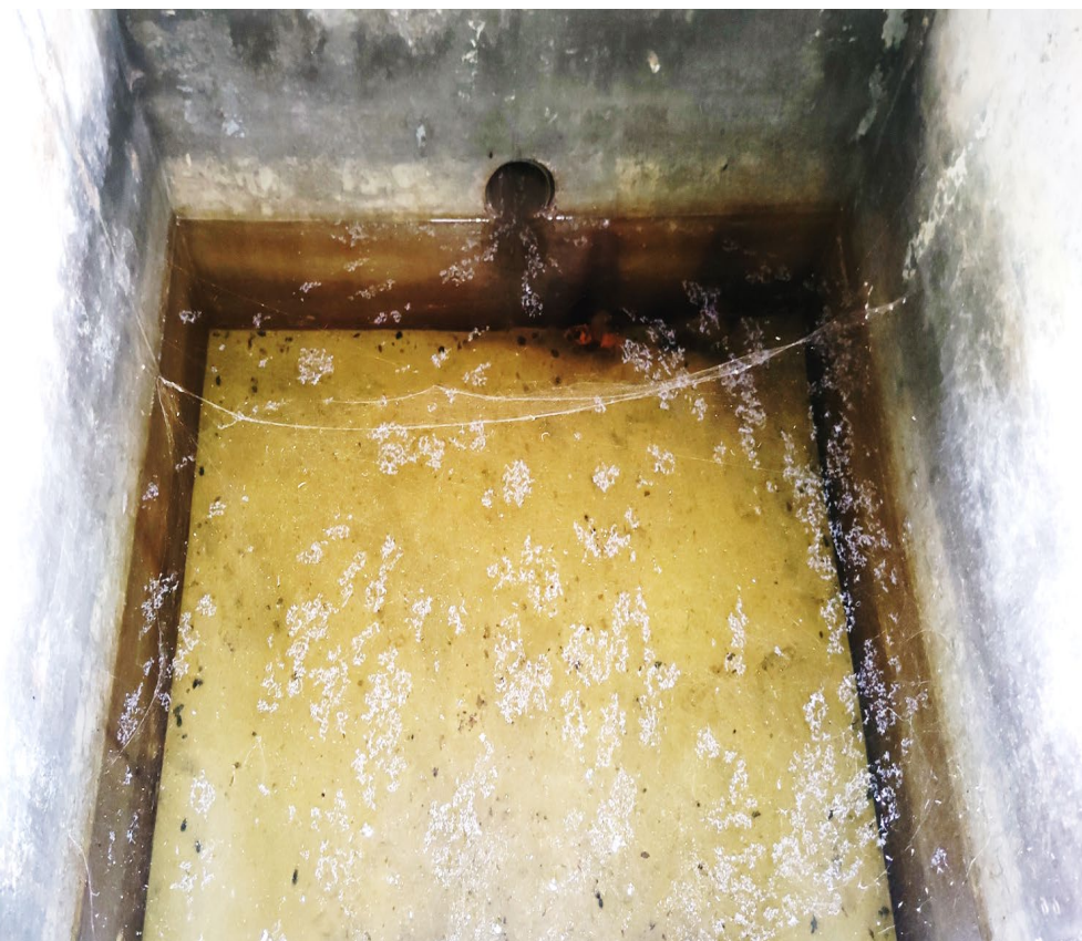
(28) Leak detection tell-tale pipe underneath the storage tank opens out to a collection chamber
